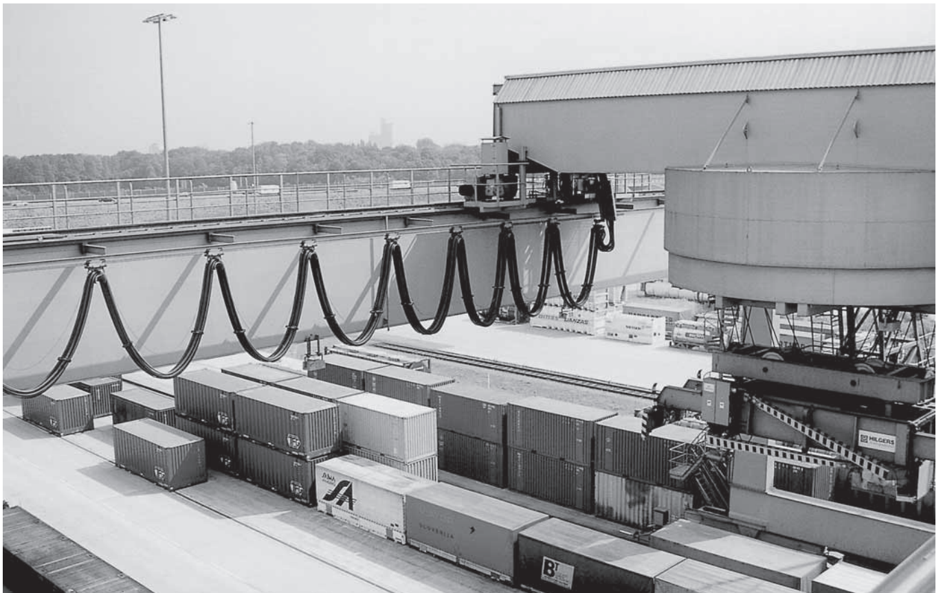
Cable carrier at a container crane
